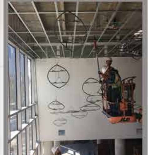
December 2017: Patrick Renner and his team begin installing lilt over the grand staircase in the new Kinder HSPVA commons.
